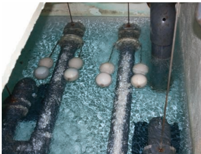
Photo 2: Gravity drainage system collector tank.
